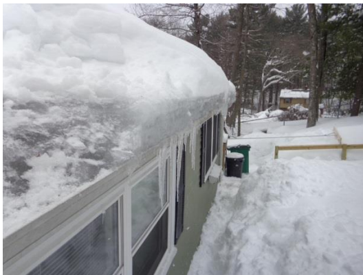
Exterior Ice Dams Leak into Houses
