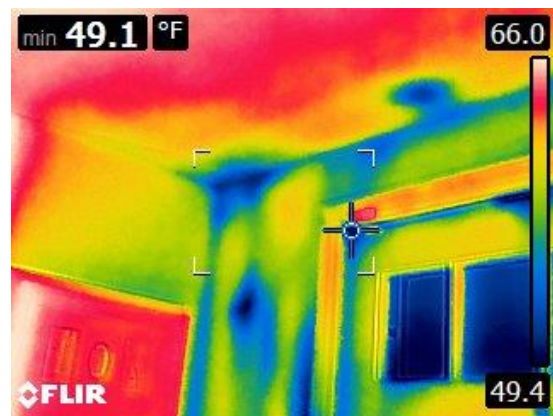
Water leak (blue) into Basement
